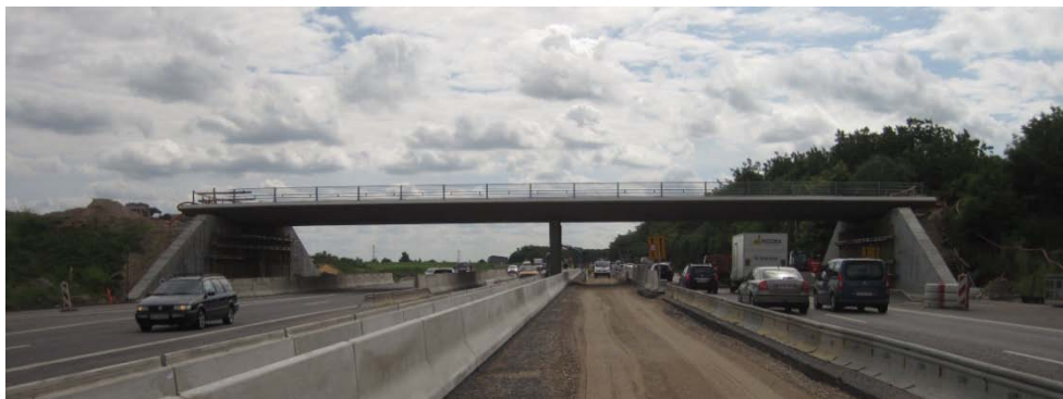
Photo showing the bridge viewed from the motorway, shortly before the new bridge was finished.
